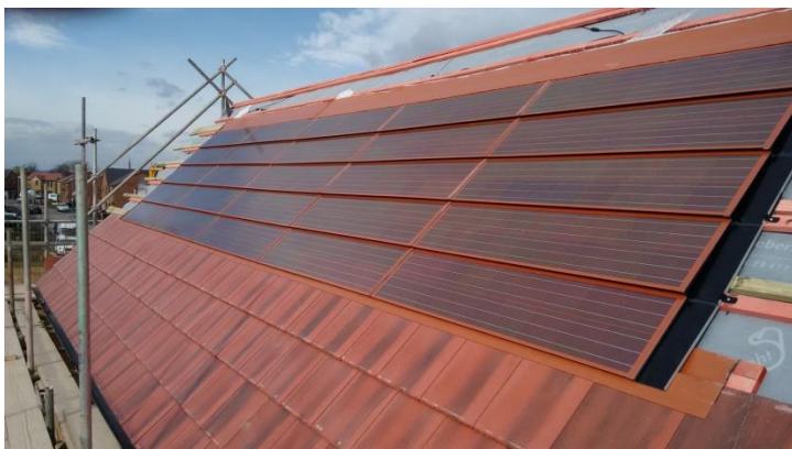
Fig. 36: Solar panels blend with roof tiles
