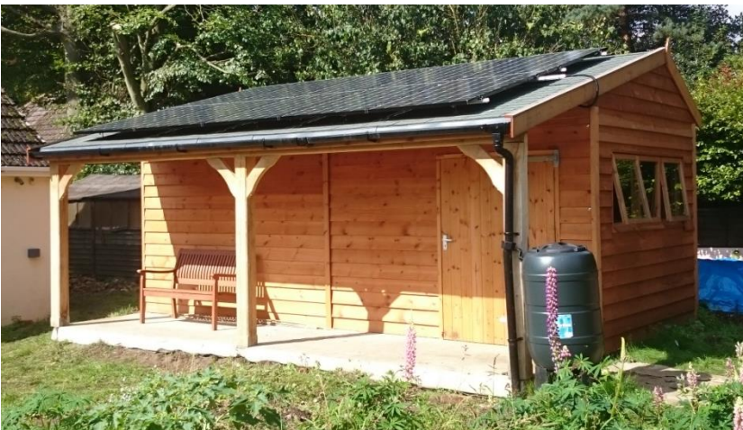
Fig. 39: Solar panels on an outbuilding are less obtrusive
